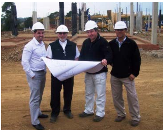
Left to right: Progress on the new Methodist seminary is on schedule. Pictured at the site are quantity surveyor Chris Venter, seminary president Ros Olivier, structural engineer Alistair Chrystal, and site manager Dereck Karvey.
